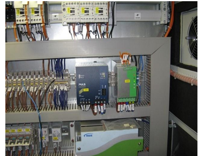
Top box of the main control
