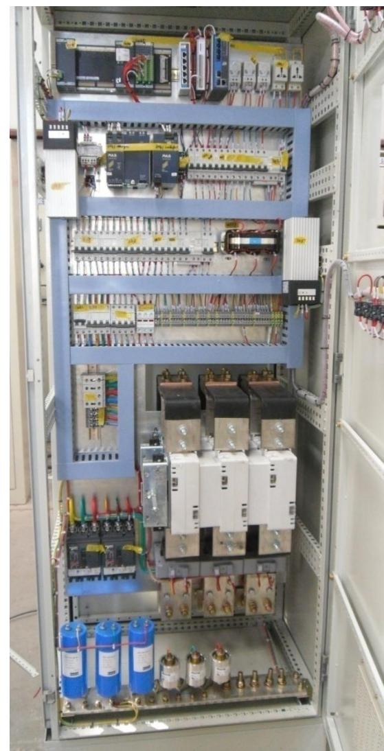
900kW main control
