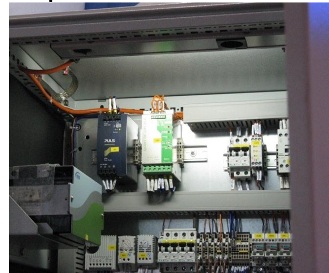
Bottom box of the main control
